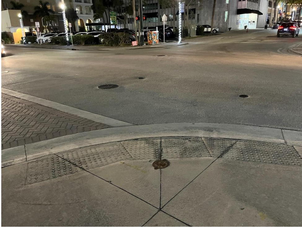
Exhibit 32: Missing ADA Compliant Sidewalk
